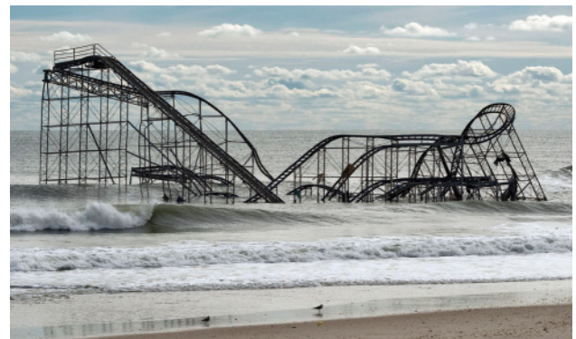
Aftermath of Hurricane Sandy, New Jersey, 2012. Global climate stability is a collective good.
